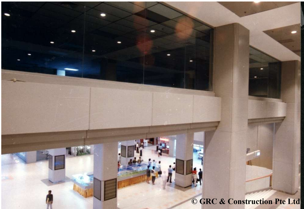
A & A WORKS AT WORLD TRADE CENTRE GFRC FALSE COLUMNS & PARAPET WALLS
